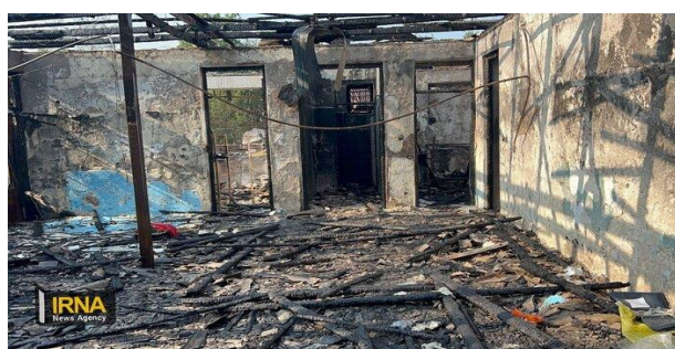
Figure 1. Interior view of the addiction treatment facility following the fire, illustrating extensive structural damage to the building. Source: Islamic Republic News Agency (IRNA), 3 November 2023. Reproduced with attribution in accordance with IRNA's stated website reuse policy.
